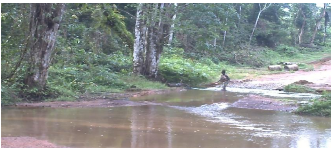
Figure 2 A view of a segment of the Nyonbeh Town-Wheasaye (Grand Kola) road awaiting the installation of culverts.
